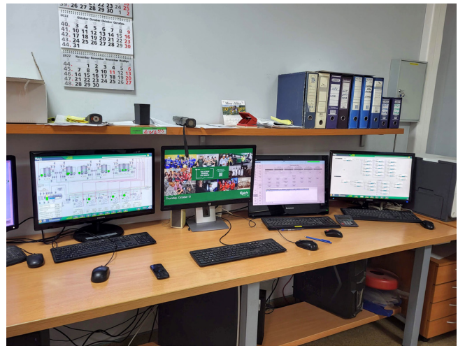
Energy management and cooling systems.
